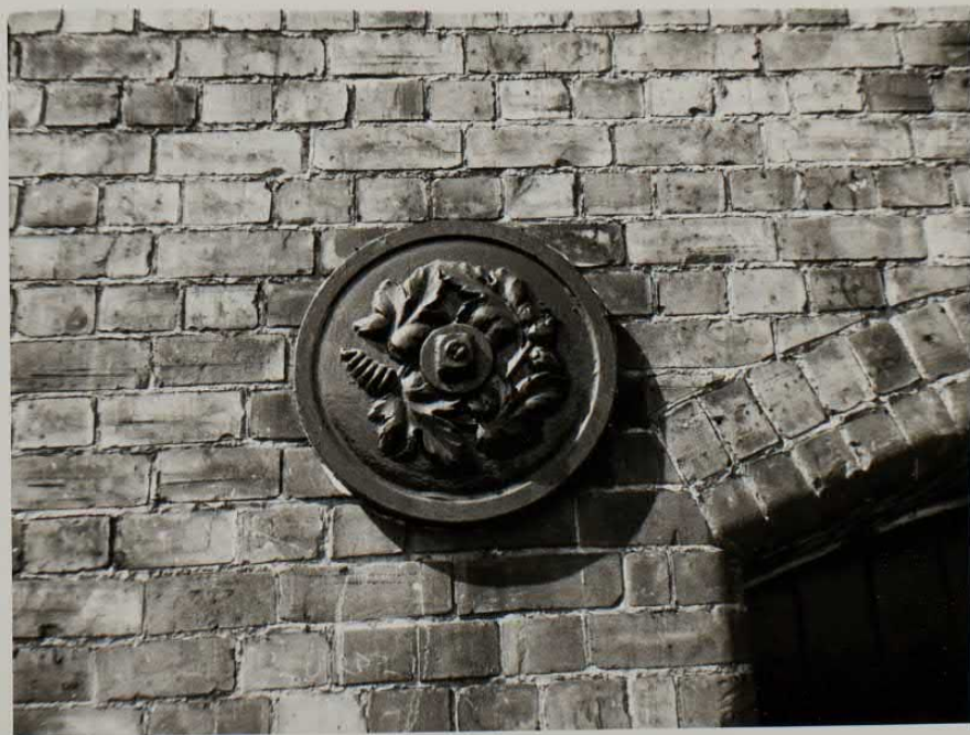
Wallplate on No 1 malting 1979
