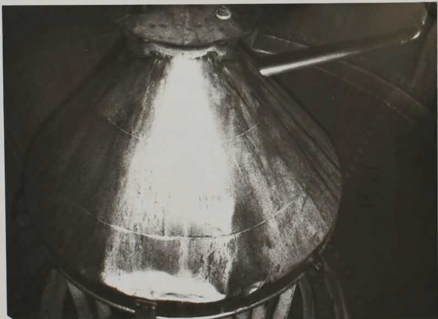
Casing over steam heater in wort copper
