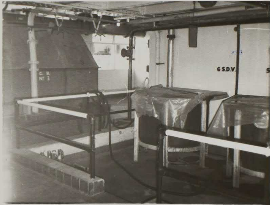
Grist bin in background and mixing vessel
