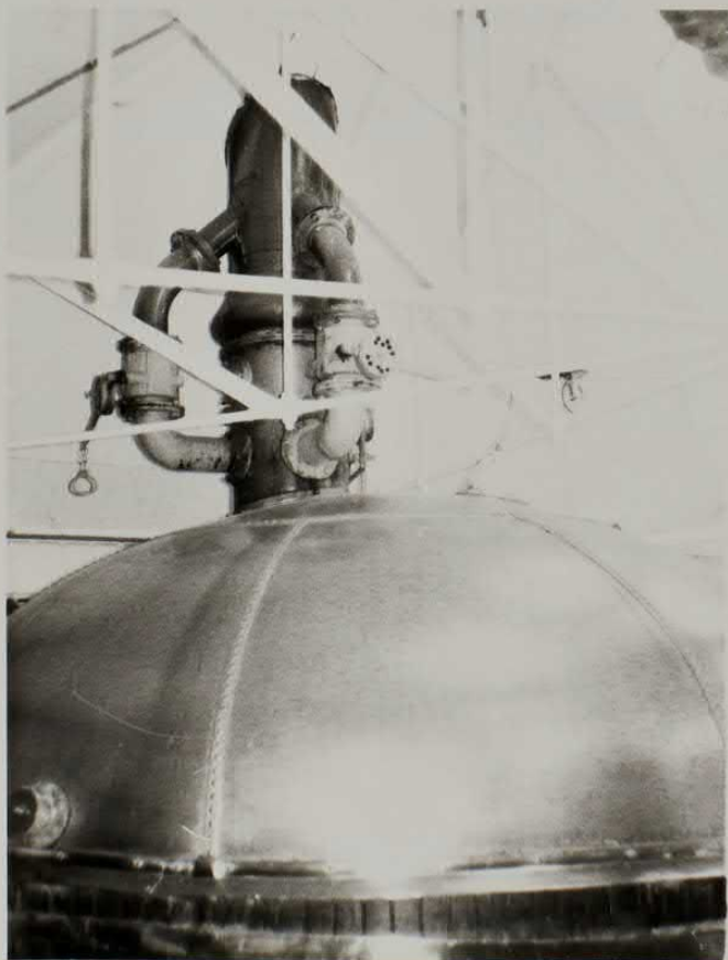
Top of Wort copper showing vent valves
