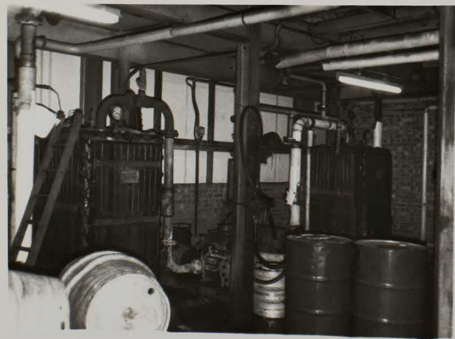
Cask washing dept. steam heated calorifiers for hot water. Storage tanks situated above
